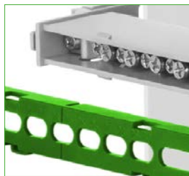
terminal strips PE + N in the bracket
